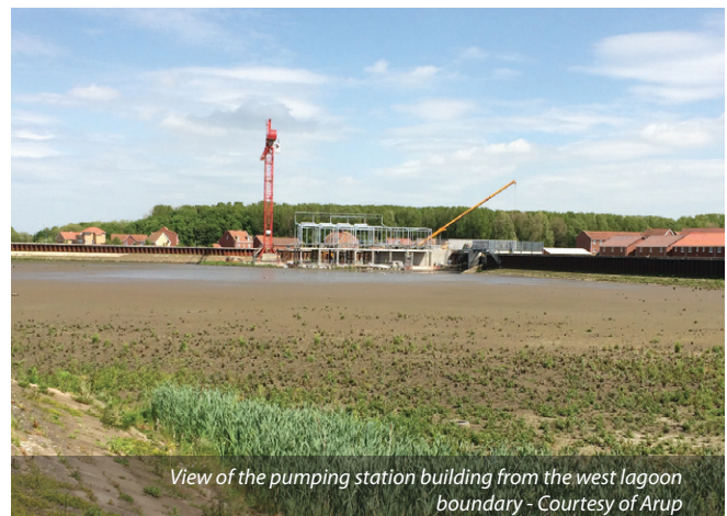
View of existing SWPS - Courtesy of Arup
